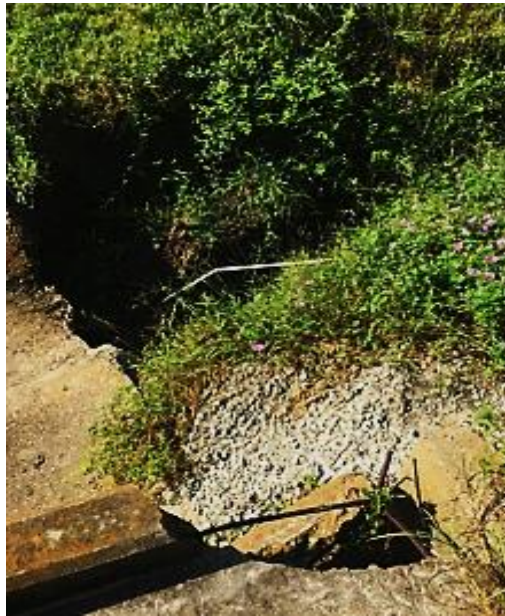
Figure 12. Erosion of the drainage system
