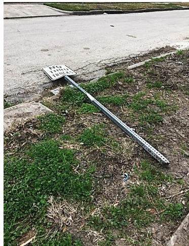
Fig 15. Traffic signs are damaged.
