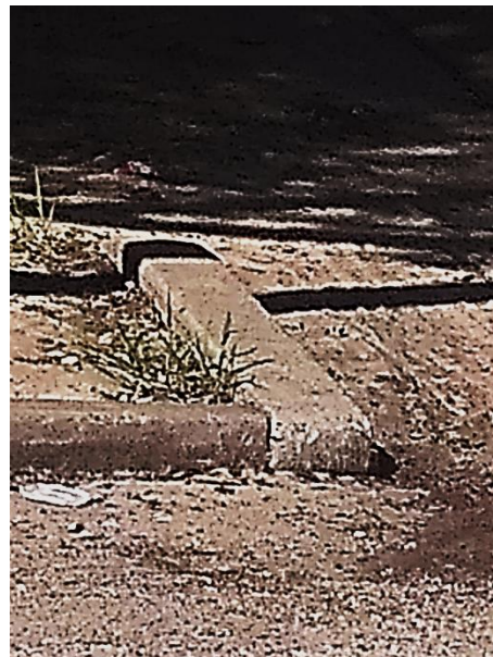
Fig 5. This curb is covered over by mud. Which makes it unusable for some. Able body occupants should take the time out to try and keep this and other curbs clear of trash and mud.
