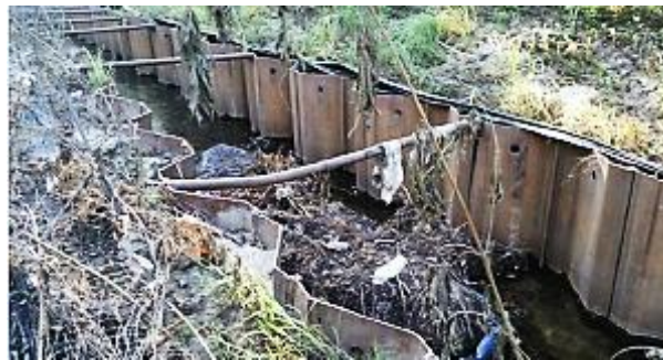
Fig 10. Plants, weeds, and debris over drainage
