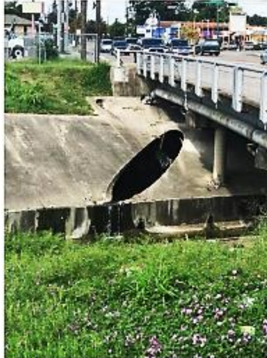
Figure 11. Holes on concrete
