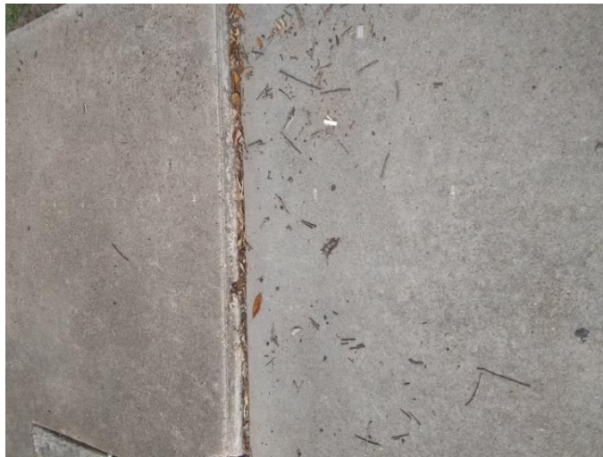
Fig 3. Uneven section of sidewalk is un-passable for some elderly and those that are wheel-chair bound
