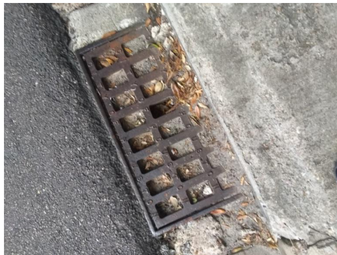
Fig 2. This sewer drain has been made useless with hard mud and debris, which might have been avoided with sidewalks to hold back the land erosions.
