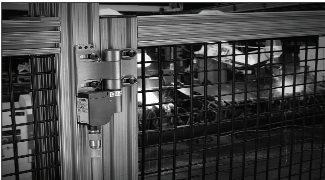
Fig 6. Interlock switch on swinging gate [7]
