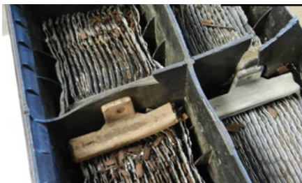
Figure 1: Two-year old battery that exploded, causing personal injury by acid burns [Roberts, 2013]
